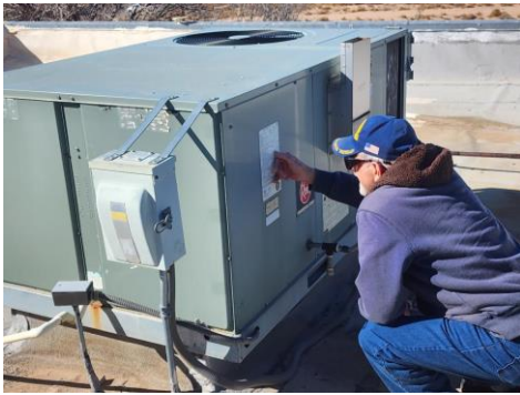
Bill Shanklin checking the HVAC specs.
